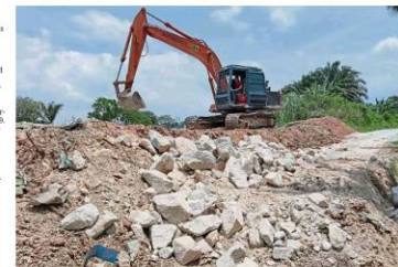
Work is taking place to strengthen the bank along Sungai Langat with rocks at Kampung Rivokul Hijau, Dengkil.
